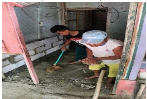
The Students Join with The Workers to Give The Mixture of Cement and Sand in The Floor (16 March 2016)
